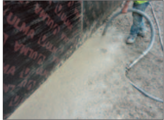
Immersion vibration of RCC without grout (IVRCC) at the Enciso dam in Spain, in 2011, which was first developed by F. Ortega at De Hoop dam in South Africa.
