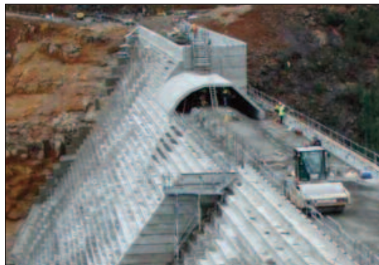
Precast concrete elements at spillway crest of Meander RCC dam in Tasmania, Australia, referred to by Brian Forbes.
