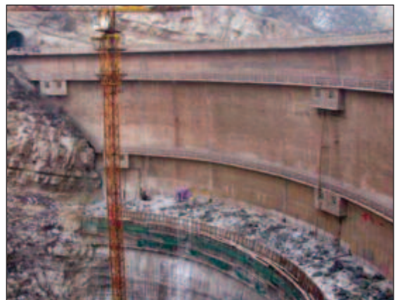
The rockfilled concrete (RFC) technology that was used for the reinforcement works of the 69 m-high Hengshan arch dam in China, as discussed by Dr Jia Jinsheng.
